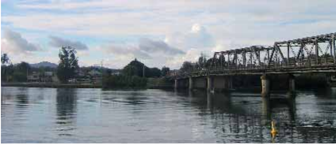
The bridge is set in a striking river landscape where the naturally vegetated coastal ranges are visible in the distance
