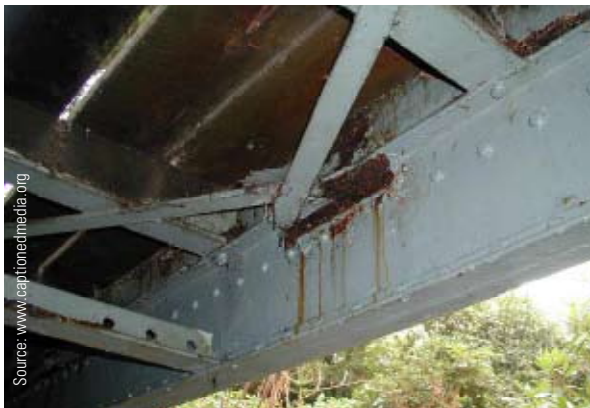
Figure 5.1: Example of corrosion caused by electrolysis
