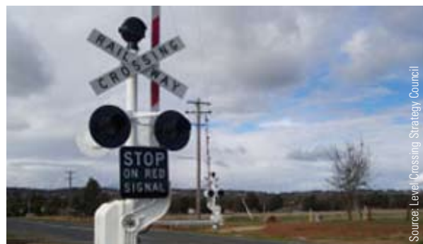
Figure 5.4: 'Active protection' at a level crossing
